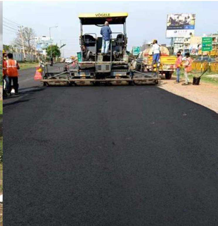
Construction of roads with recycled plastic waste on the Athaang Devanahalli Highway
