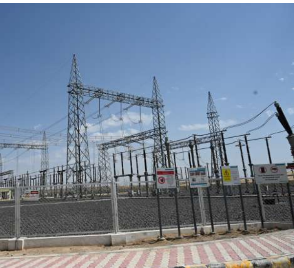
Ayana's solar plant unit substation
